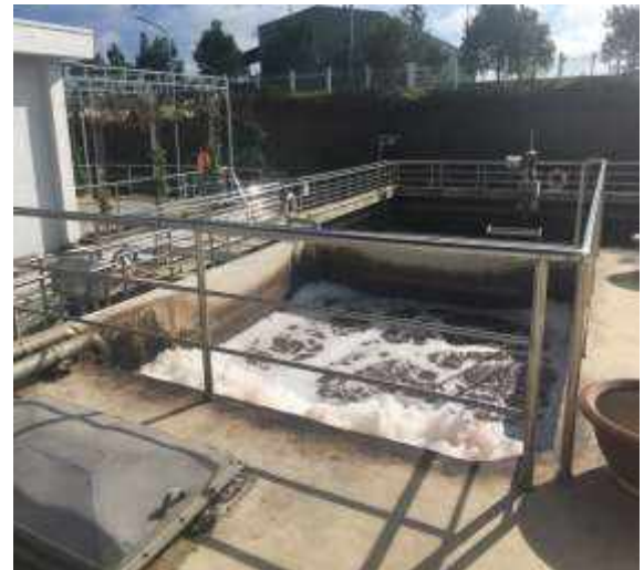
Bể trung gian
